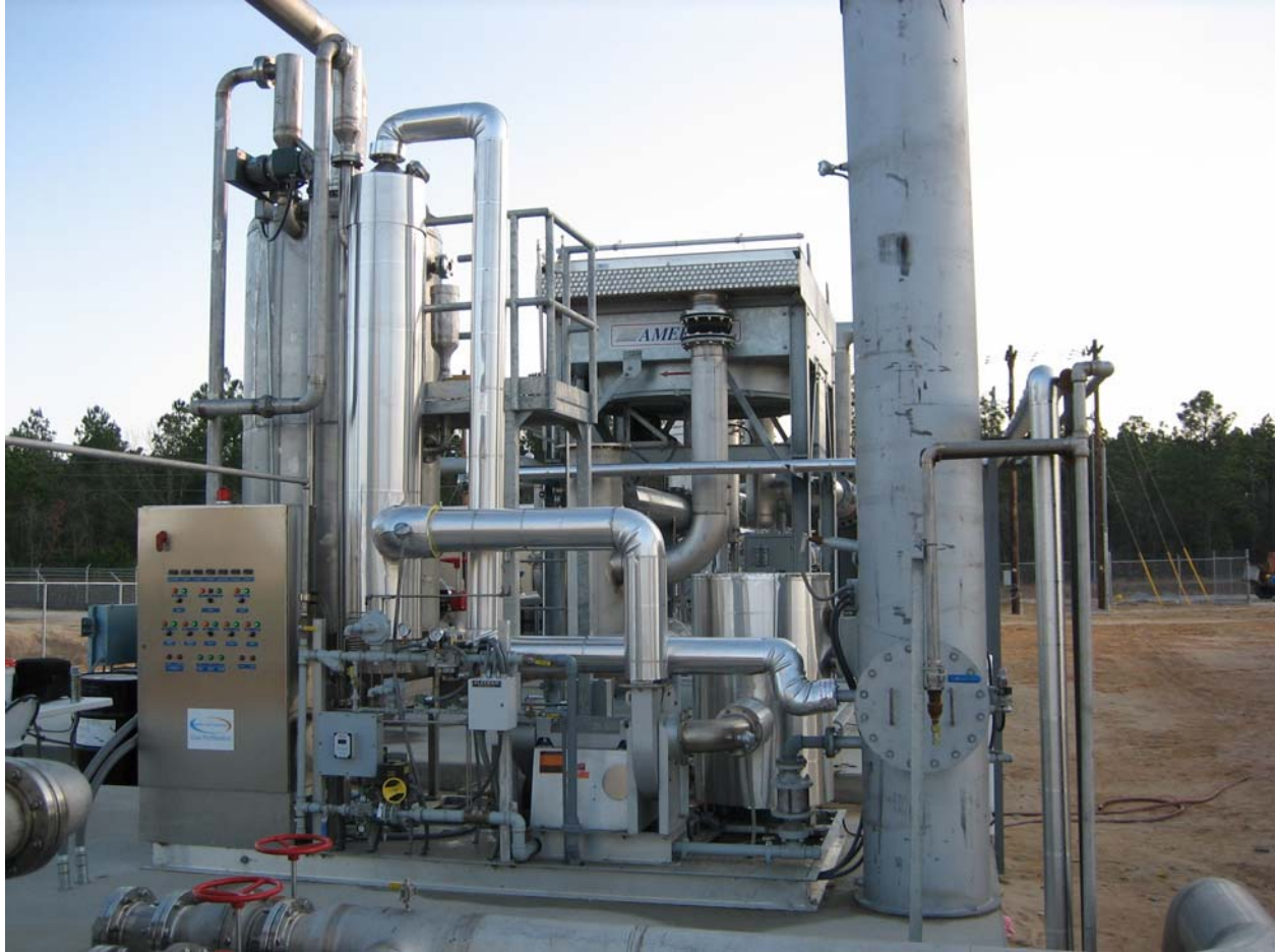
Picture of 2,500 SCFM SWOP™ System at site in South Carolina
