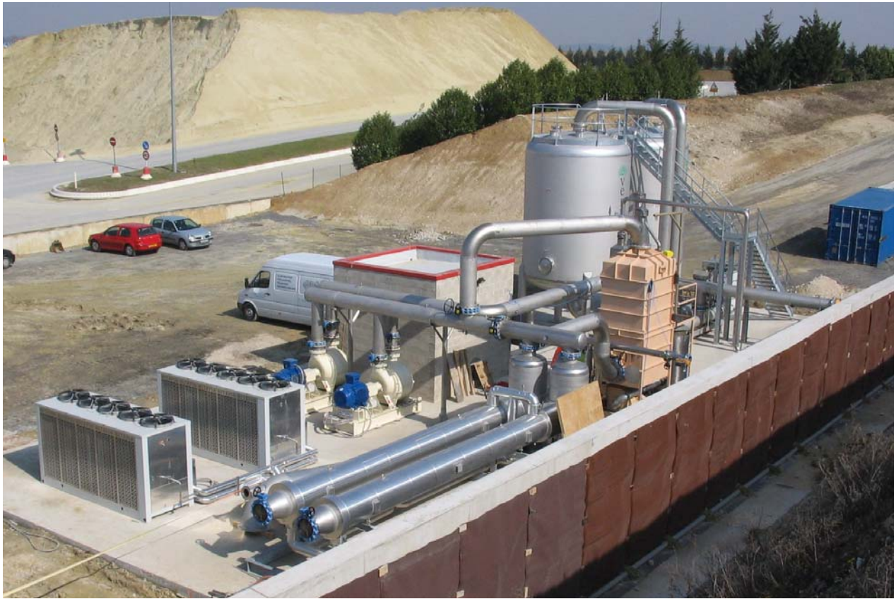
Complete landfill gas treatment package at Paris landfill (ground flare not shown). (Note that all piping had not been installed at the time the picture was taken)
